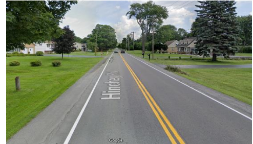
Typical Pavement Condition
